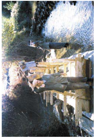
In the Wadi Khalid area of North Lebanon, along the Syrian border, a small water dam is constructed with help from CHF International.
